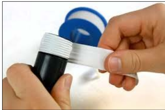
Securing the connection between the water flow meter and BNC pipe connector using thread seal
