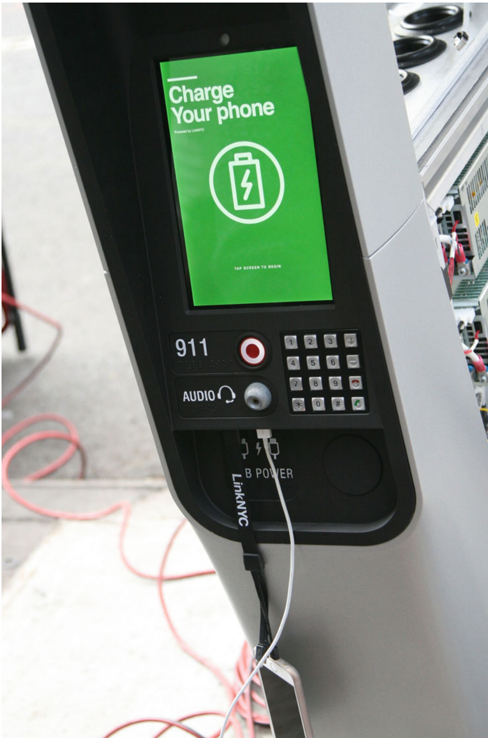
Figure 13-18. Link station being set up; the kiosks offer phone charging, Internet browsing, free phone calls, and emergency services calling
