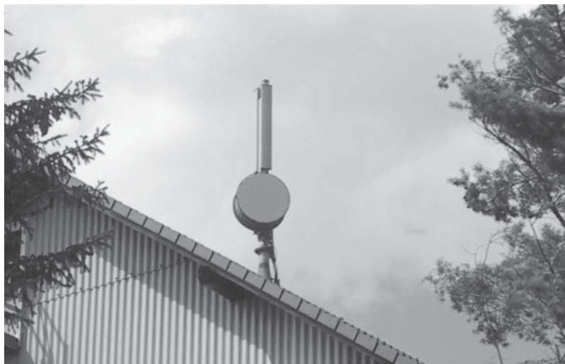
Figure 1.20 A typical antenna of a GSM base station. The optional microwave directional antenna (round antenna at the bottom of the mast) connects the base station with the GSM network. Source: Martin Sauter. Reproduced by permission of Martin Sauter
