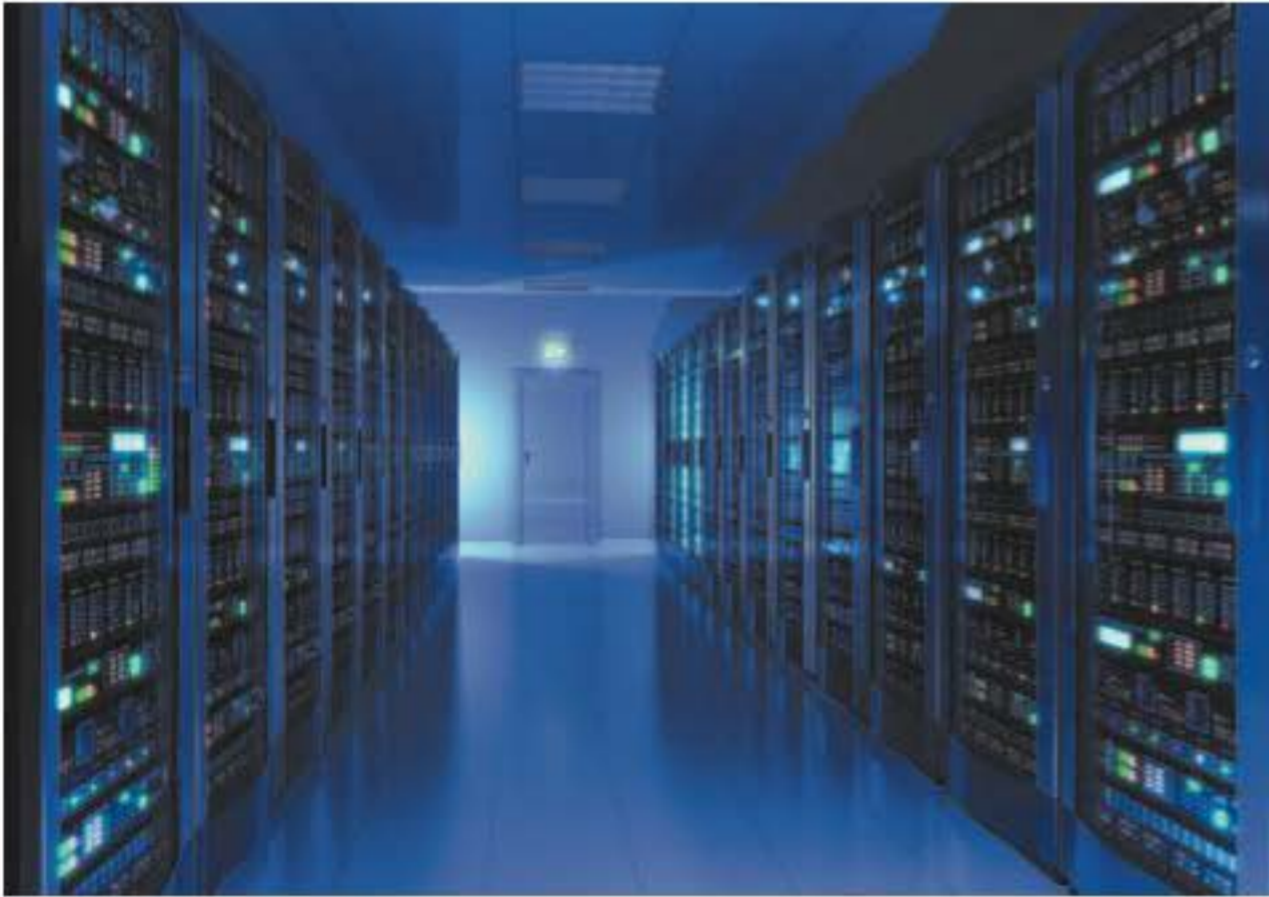
FIGURE 12-37 The rapid growth of data centers and server farms has increased energy consumption significantly and raised environmental concerns.
